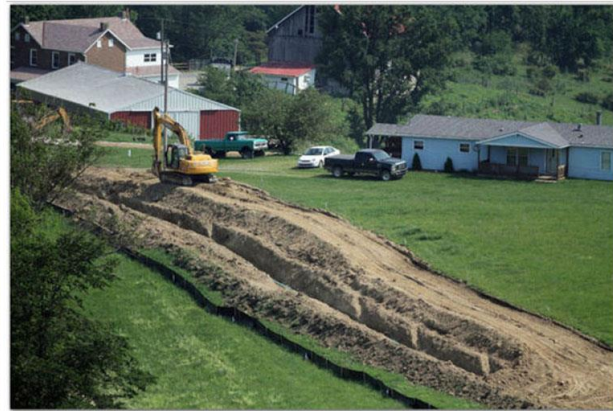
A pipeline laying operation near a home in Greene County. ( Michael Bryant / Staff Photographer )
